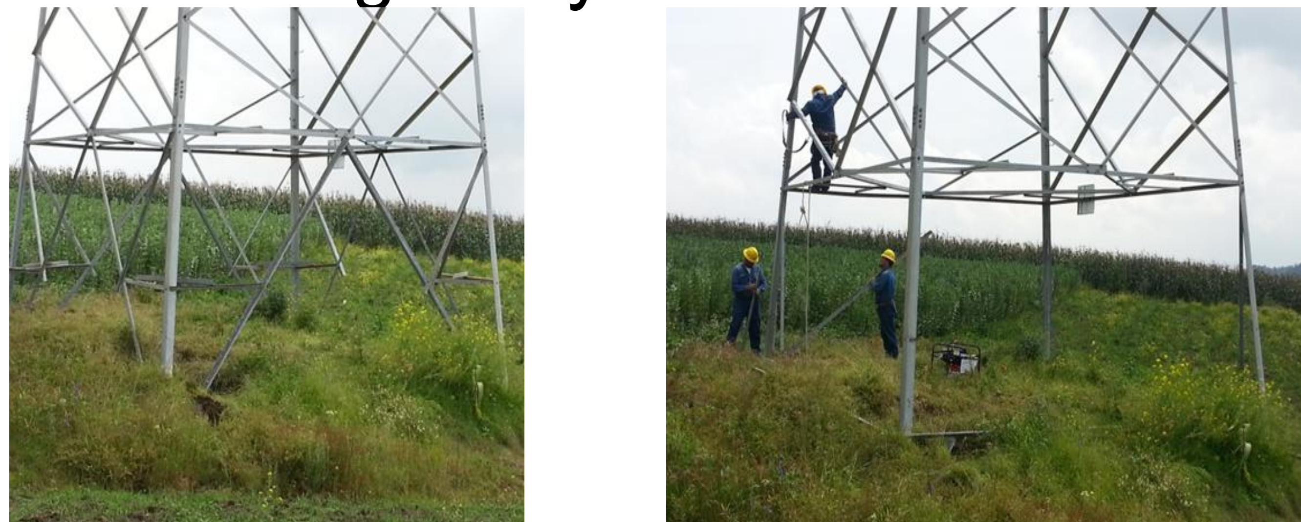
Figure 1. Transmission line tower with and without redundant members in the bottom panel.
