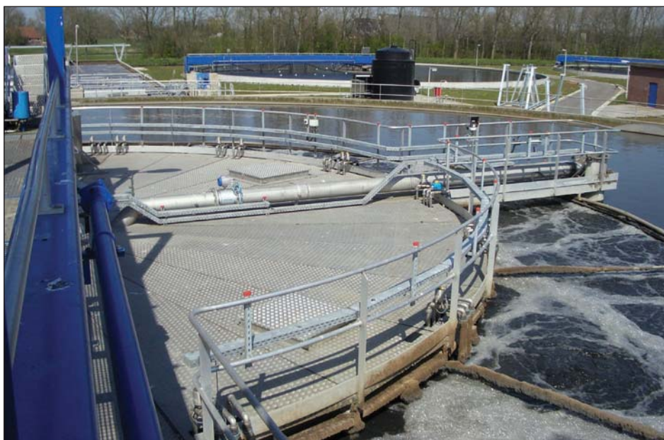
Figure 1: The modeled clarifier tank in the wastewater treatment facility. Photo courtesy of Witteveen+Bos.
