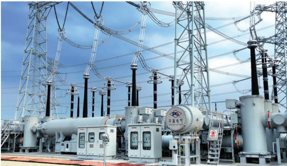
Figure 1. 1100-kV GIS. Image courtesy of Pinggao Group.
