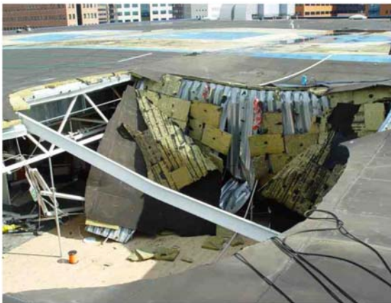
Figure 1. The damage of the roof.
